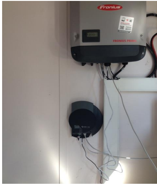
Figure 3. Solar-log device and on grid inverter
