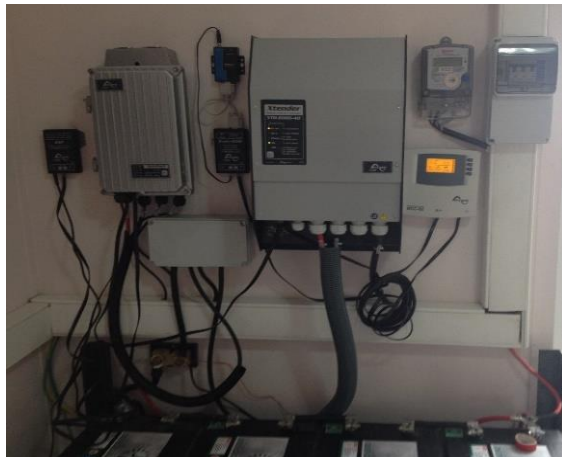
Figure 4. (b). Off Grid Inverter (Studer)
