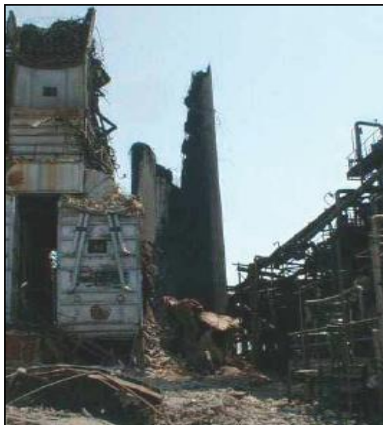
Figure 8. 115 meters high collapsed Tüpras Refinery RC Chimney
