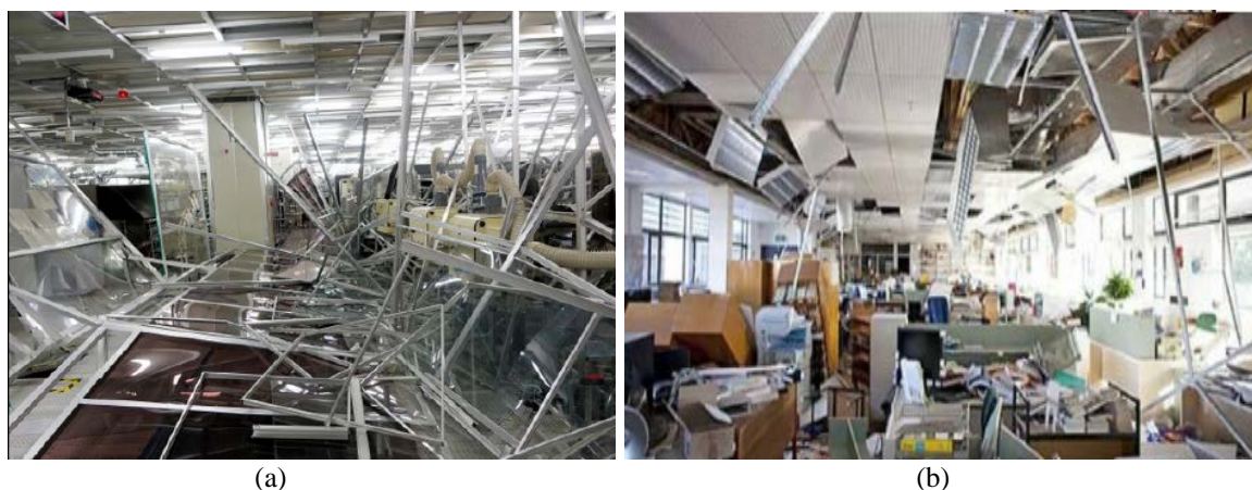
Picture 1. This picture is an example of business offices that have prevented the operation after the earthquake. Pictures (a) and (b) show the Sony Kumamoto sensor factory damaged in the earthquake in Japan in April 2016.
