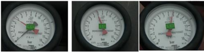
Fig. 5. Pressure change control in other tanks after emptying tank
