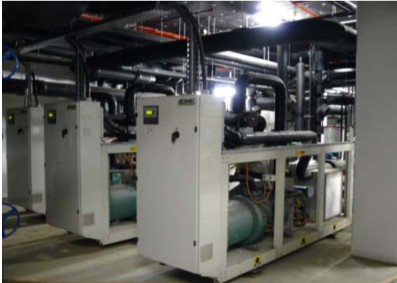
Figure 11. The heat pumps
