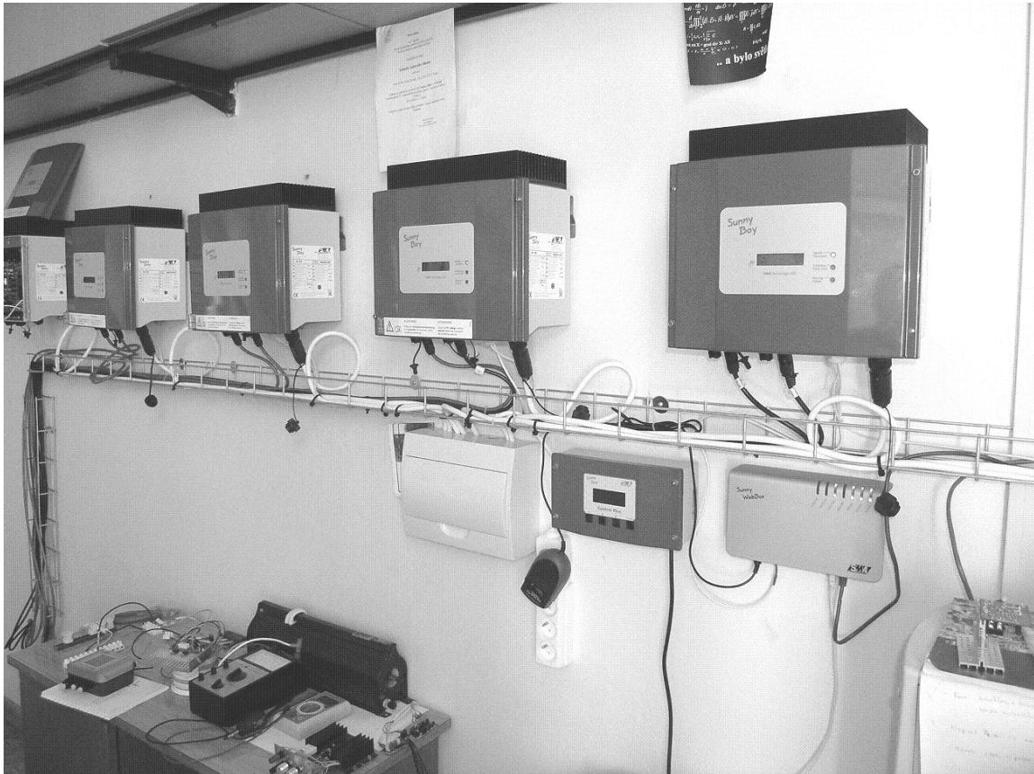
Figure 3. Data logger, switchboard and Sunny Boy inverters placed in the laboratory.
