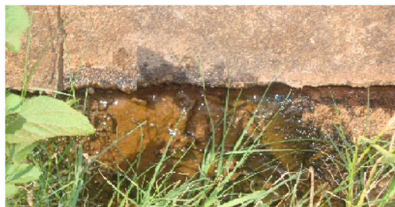
Figure 3. Irrigation water leaking through a cracked delivery canal lining
