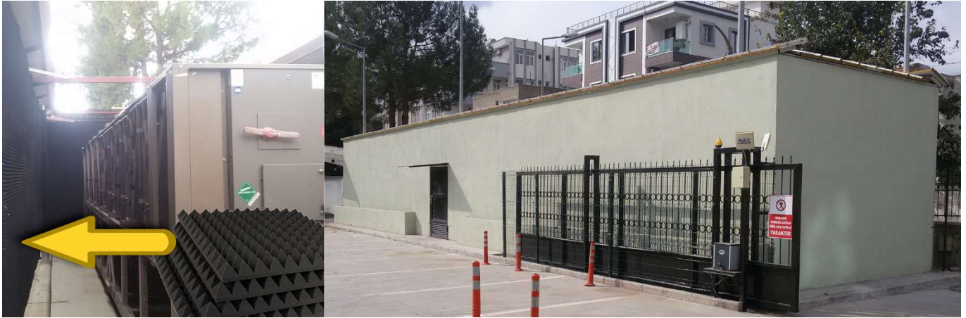
Figure 2. Isolation room for air-cooled liquid chiller noise
