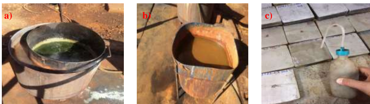
Figure 4. a) Acid tank b) Rinsing tank c) Surface cleaning
