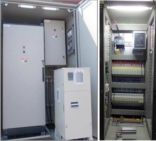
Figure 10. Automation panels of distribution center a) RTU, DCU and rectifier b) EQA in the panel.
