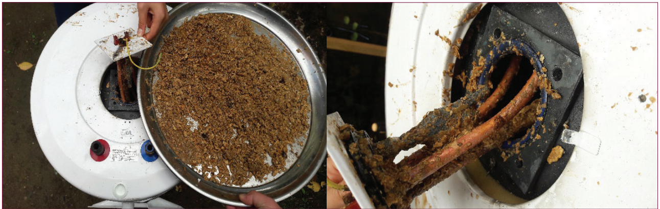
Figure 2. Sampling of LS in domestic boilers operating at temperatures (60-75)°C.
