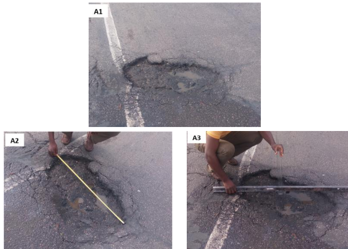
Fig. 3 Pothole and Measurement of Severity Level
