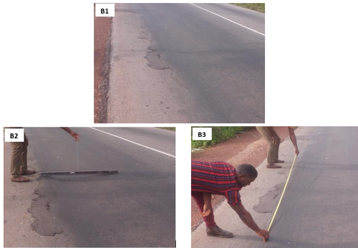
Fig. 4 Rutting and Measurement of Severity Level
