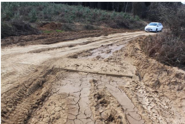
Figure 4. Culvert completely covered with sediment
