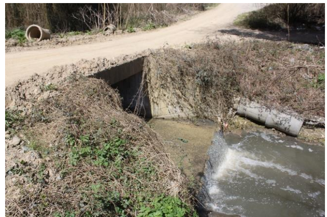
Figure 5. Completely open seventh culvert
