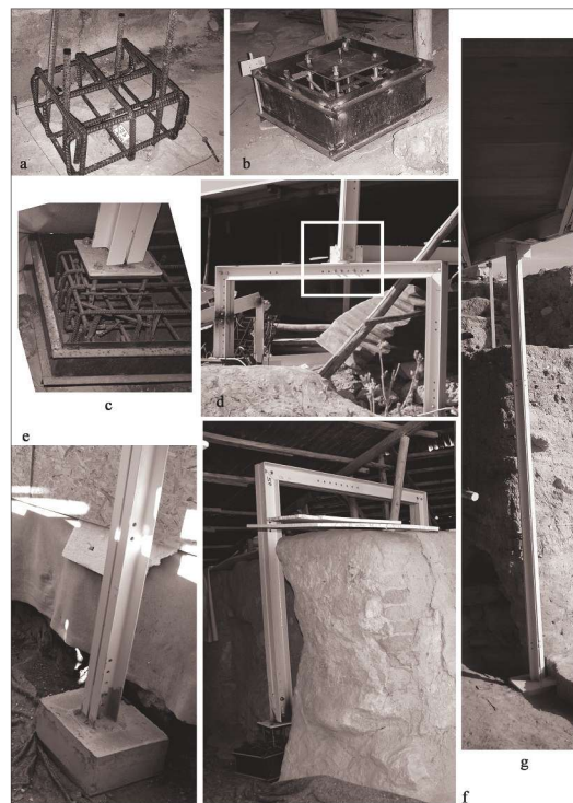
Fig. 2. Arslantepe, Details of the metal structure sustaining the roof. a-c and e: basement system. d and f: metal 'bridges' supporting the vertical posts. g: simple vertical pole at the edge of the protected area
