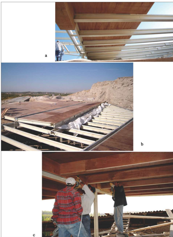
Fig. 5. Arslantepe, a and b: the roof-covering wooden boards. c: lining the metal beams with wood.
