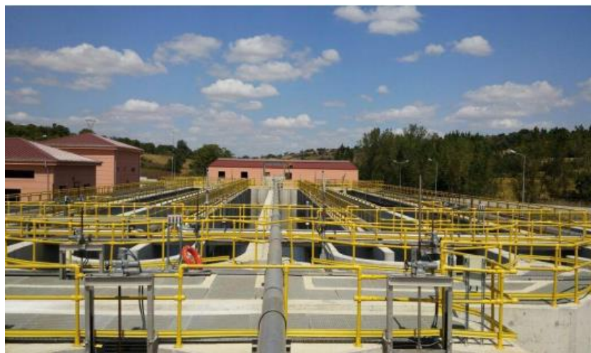
Figure 2. Malkara Advanced Biological Wastewater Treatment Plant
