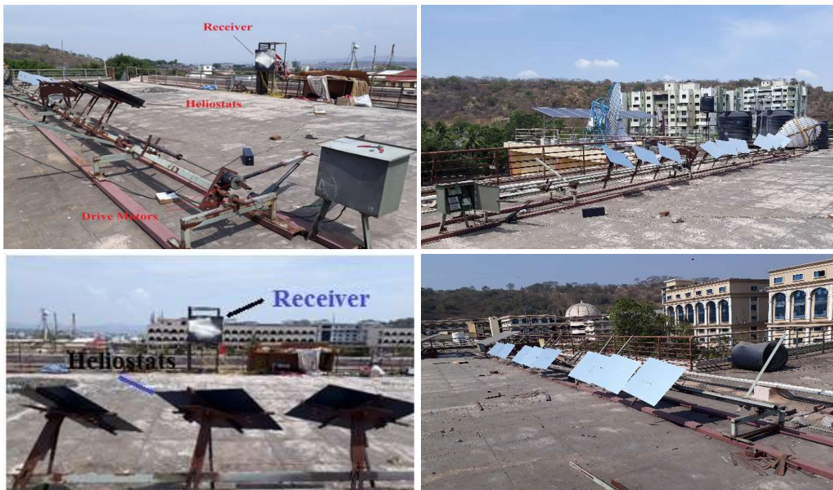
Figure 1. Heliostat system and the receiver plate [Location: Pune, Maharashtra, India] (photographs from different angle)
