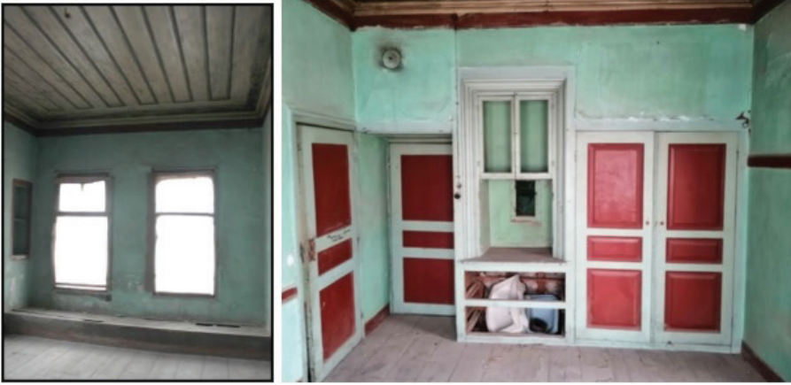
Fig. 28: Timber bench and the cupboard used as a closet in room Z04. (By Karakuş, 2020)
