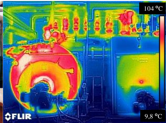
Figure 4. Thermal image of boilers and steam distribution lines
