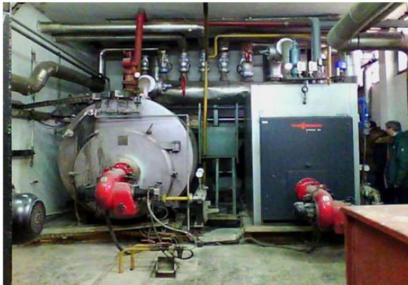
Figure 3. Two steam boilers installed in the boiler house
