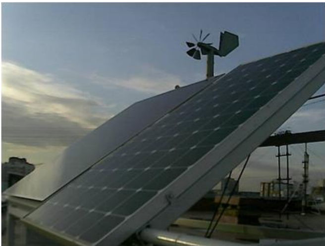
Fig. 1. Solar panels installed in Ufa State Aviation Technical University
