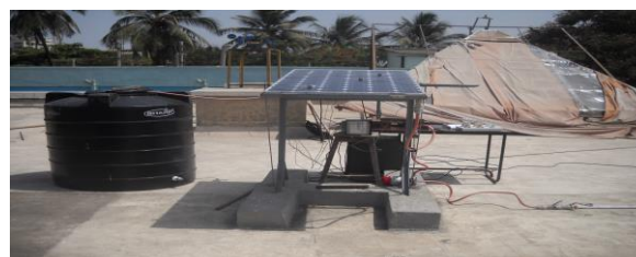
Fig. 2. Experimental set up of hybrid (PV/T) solar water system with accessories.
