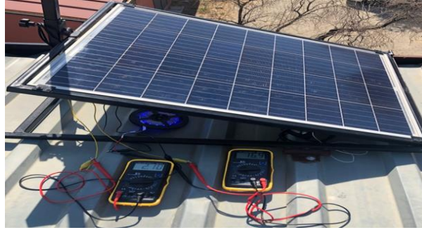
Figure 2. Polycrystalline photovoltaic solar panel.
