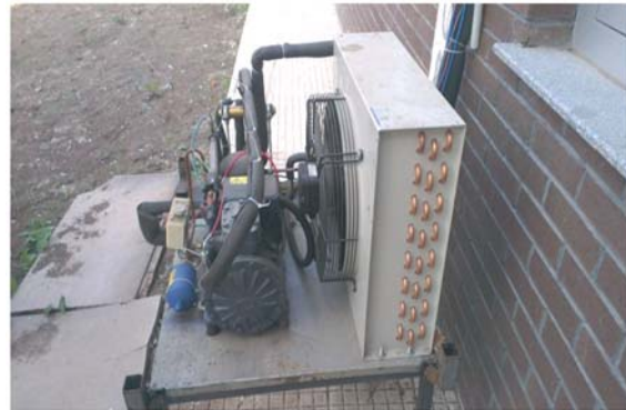
Figure 2. Outdoor unit of the ASHP
