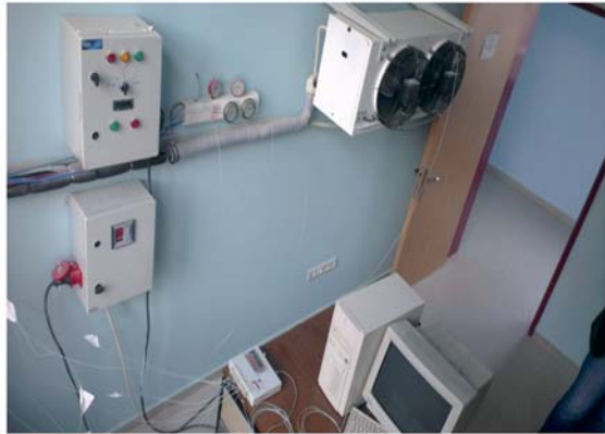
Figure 1. Indoor unit of the ASHP
