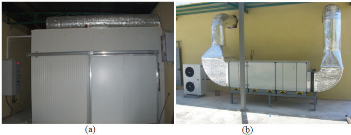
Figure 1- Experimental cold store (a) and air conditioning unit (b)
