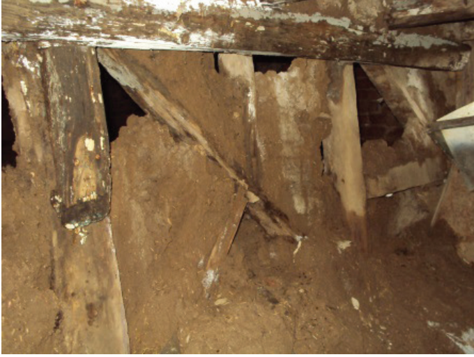
F. 19: Timber Structural Elements on the Intermediate Wall in the Basement Floor (It can be observed because of the plaster fall) (PA/18. 11. 2009)
