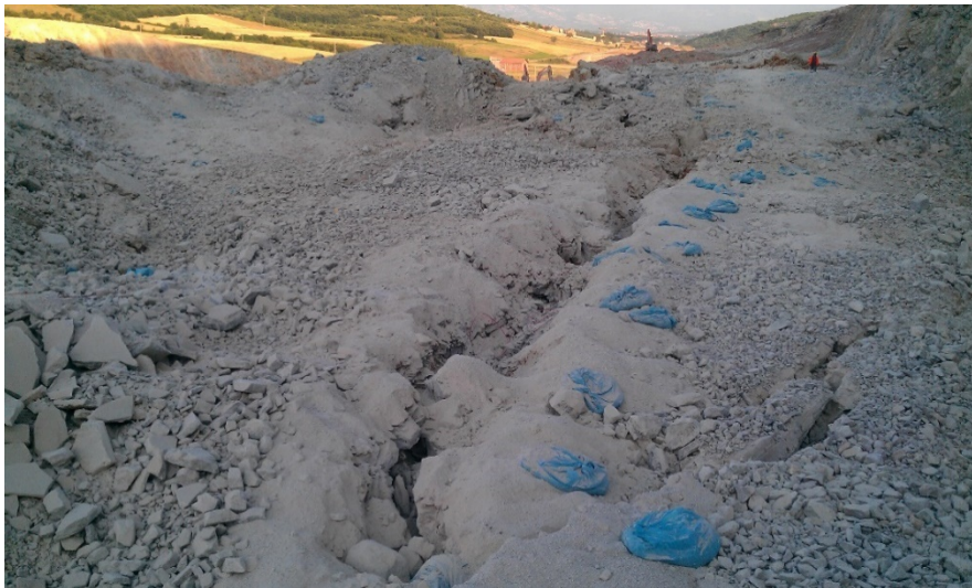
Figure 7. Damage to the bench from the impact of product blastholes - the case in Bellanica
