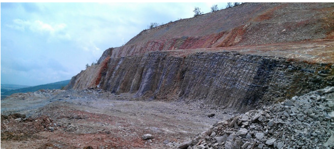
Figure 7. The view after removing the mined material of cutting the bench with contour blasting
