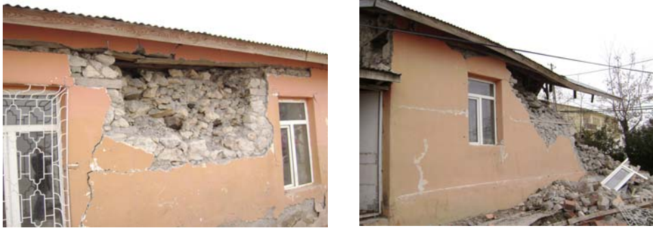
Fig. 3. Some examples of masonry failures (Original)
