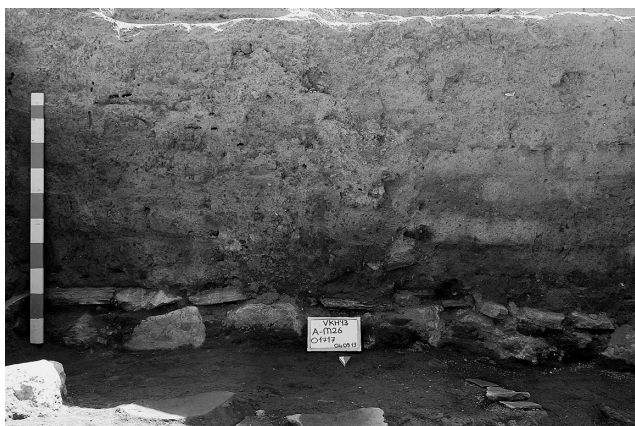
Fig. 7 South wall of the room opening to the storage area (01717). Stone foundations and brick body. Van Fortress Mound, trench M26
