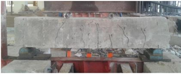
a). Fire damaged beam
