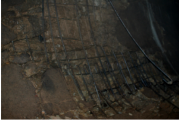
Şekil 8: Kemer betonu sol yan duvardaki donatı meydana gelen boşluk (km 6+125). Figure 8: Cavitations occurred on the left of side of the wall reinforcement of arch concrete (km 6+125).
