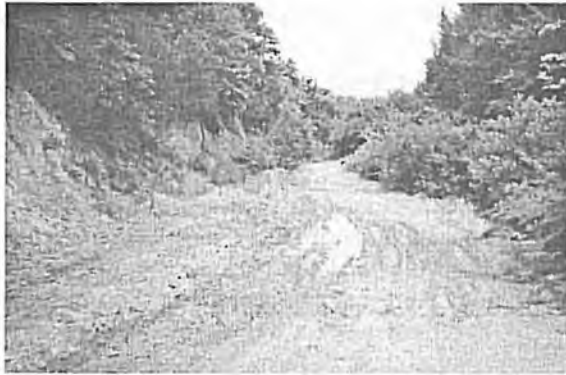
Figure 3. The conditions of 02 code forest road, ditch, and roadbed prior to pavement activities (Photo: T.Ozturk)
