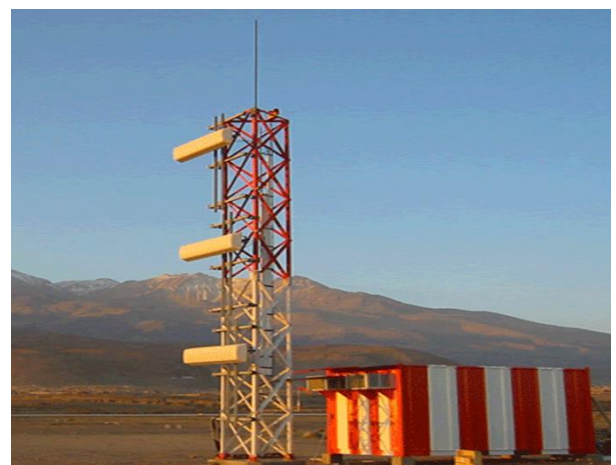
Fig. 5. Glide slope antenna [6]
