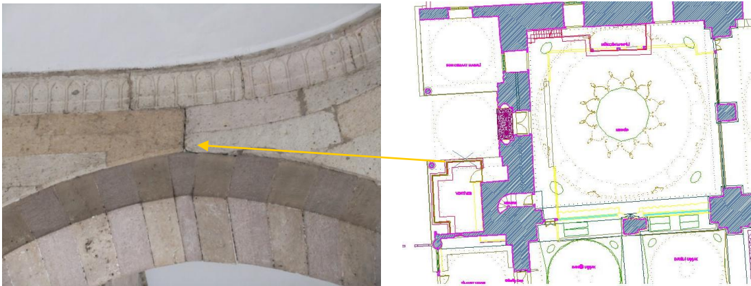
Şekil 21. Vestiye-Giriş arası kemer çatlağı (Figure 21. The crack at the arch located between the Cloakroom and Entrance)
