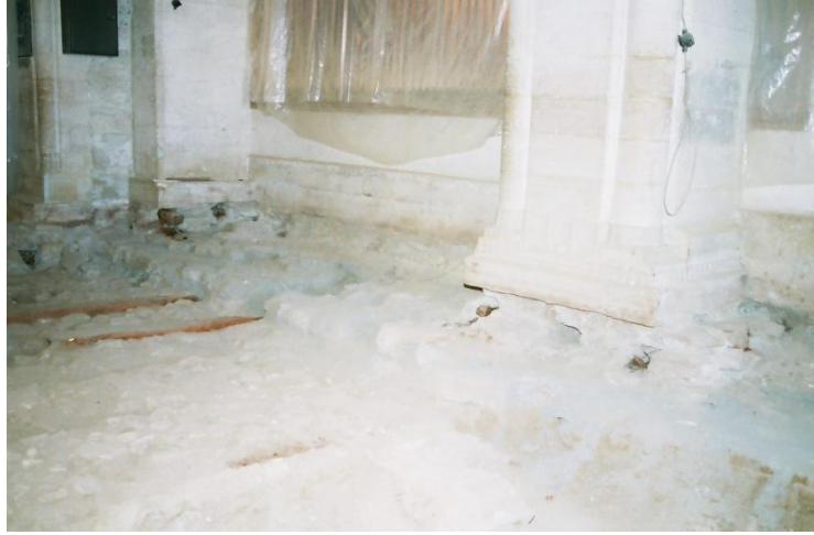
Şekil 5. Semahane zemininin kazı sonrası durumu (Figure 5. The view of the Whirling Hall ground after the excavation)
