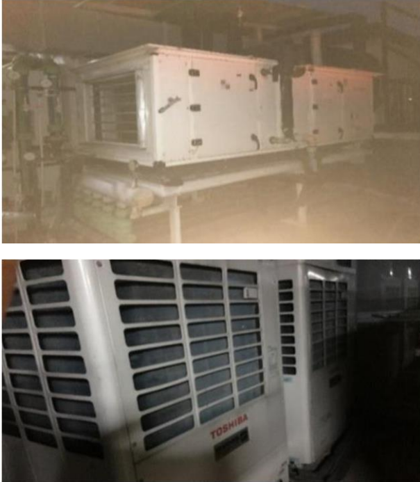
Fig. 9. Hotel enterprise ventilation and air conditioning units with energy audit
