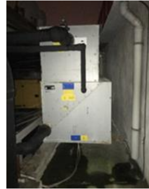
Fig. 10. Hotel facility chiller unit with an energy audit
