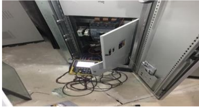
Fig. 12. Hotel management main distribution (ADP) panel with energy audit
