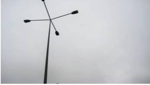
Şekil 19. (Tip 3) Dörtlü Kavşak Aydınlatma Elm Figure 19. (Type 3) Quad-Junction Lighting Fixture
