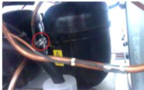
Figure 6: Thermocouple mounted on the compressor outlet pipe.
