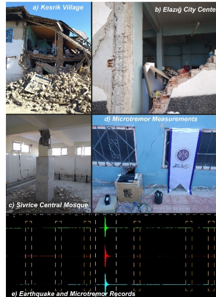
Figure The damaged structure and Microtremor measurement
