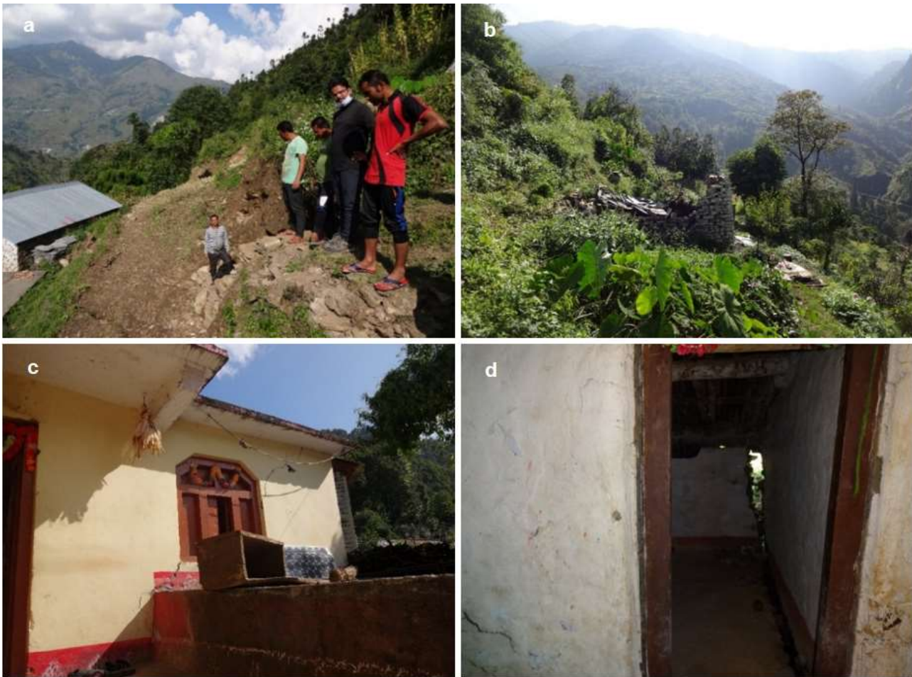
Fig. 7. Ground subsidence related damages in the Malupati Village; (a) ground fissure in agricultural fields, (b) collapsed a house, (c) crack in a house and (d) detached back side wall of a house
