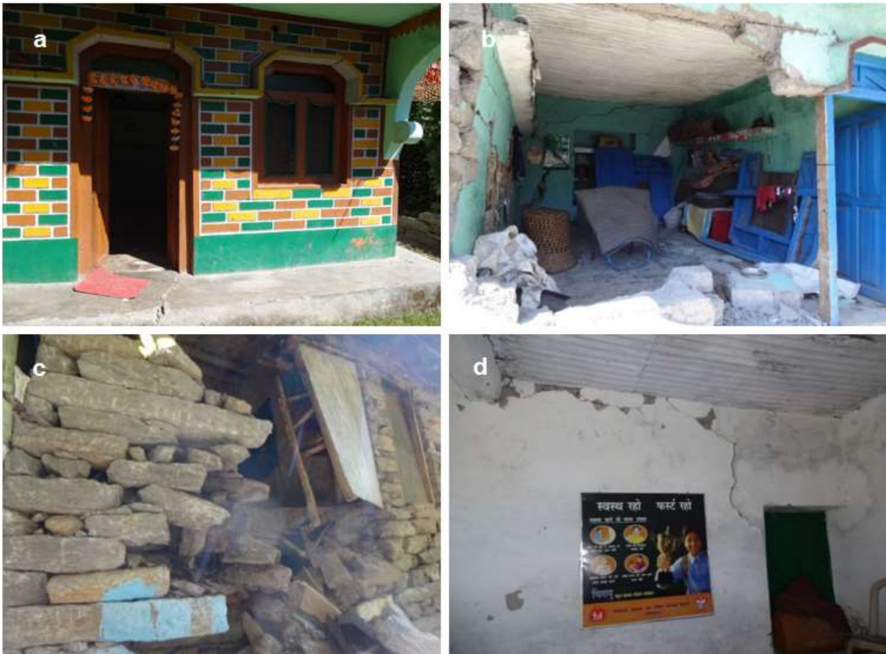
Fig. 17. Cracks in houses of Khela Village due to creep movement; (a) cracks in house at Ala Tok, (b) severally damaged house at Kolpani Tok, (c) damaged right-side wall of traditional house at Chetkala Tok and (d) cracks on roof column and wall of primary school at Chetkala Tok
