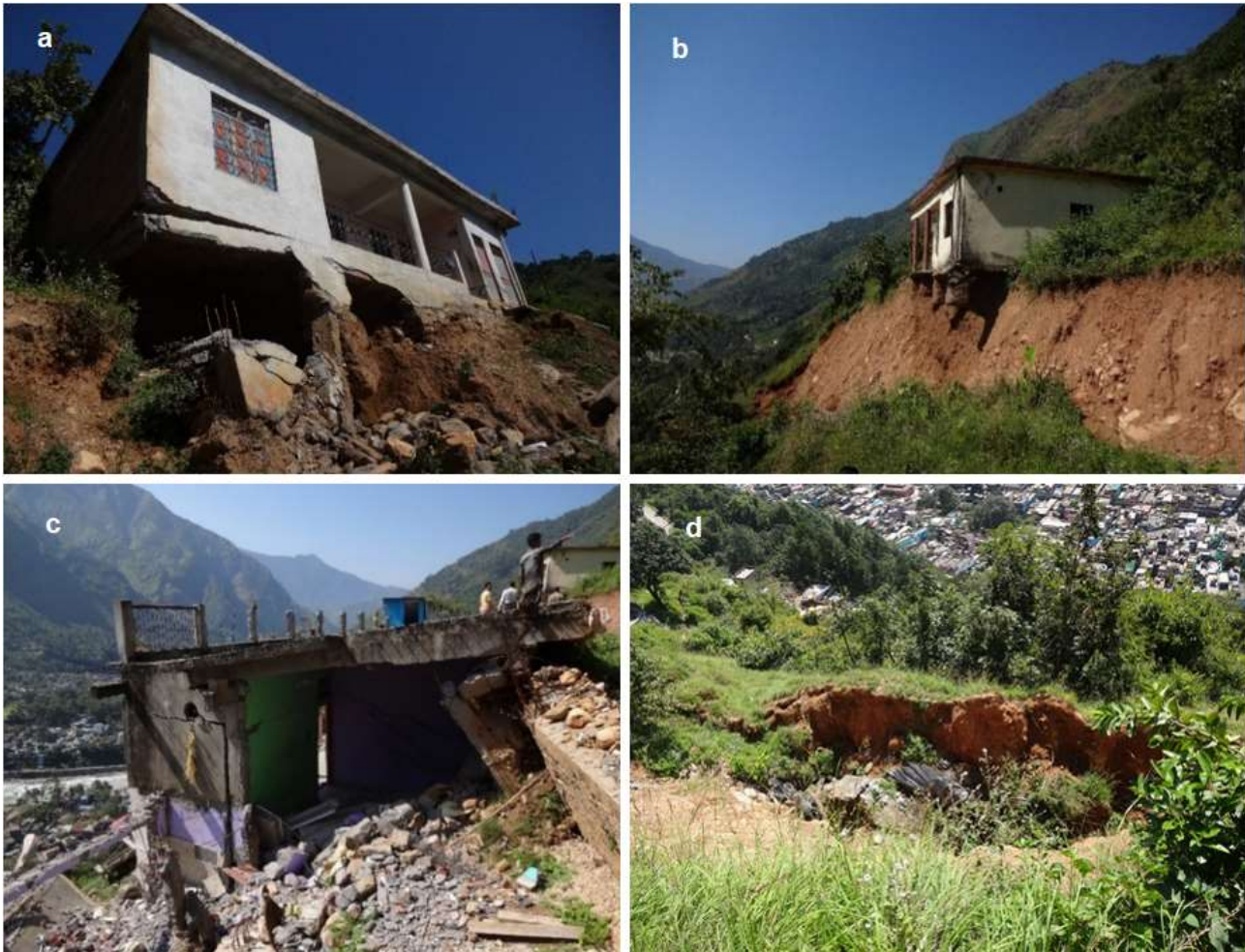
Fig. 18. Damaged structures in Gwalgaon due to subsidence in loose debris materials during heavy rainfall; (a) scoring foundation of a house, (b) hanging foundation of a house in ground fissures zone, (c) damaged house over completely subsided loose debris mass and (d) a toilet was subsided in loose debris mass and deep sink hole was formed
