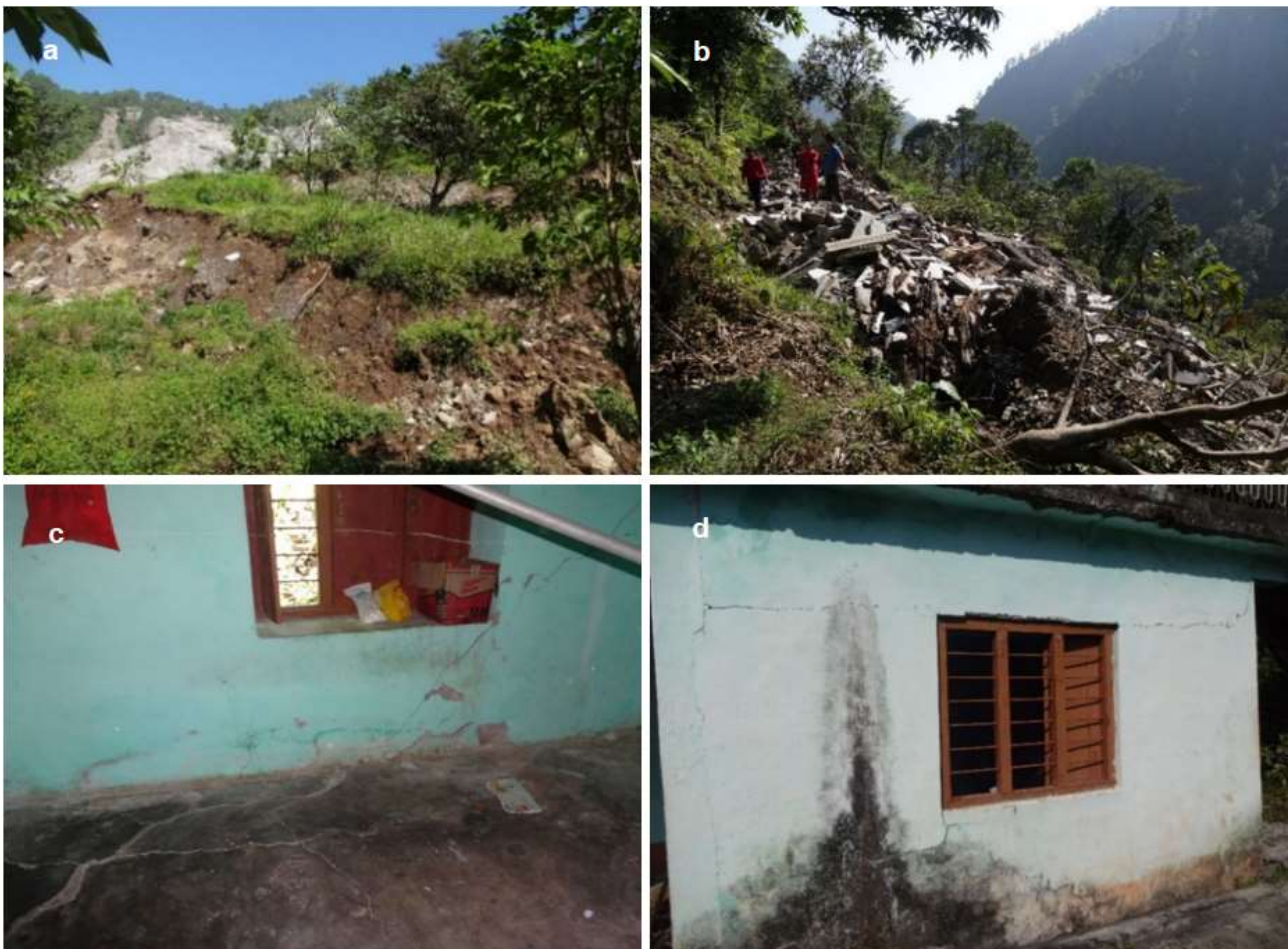
Fig. 15. Slope instability and associated damages in the Gat Tok; (a) ground fissures zone, (b) destroyed a house, (c) cracks on floor and wall of a house and (d) cracks on front portion wall of a house
