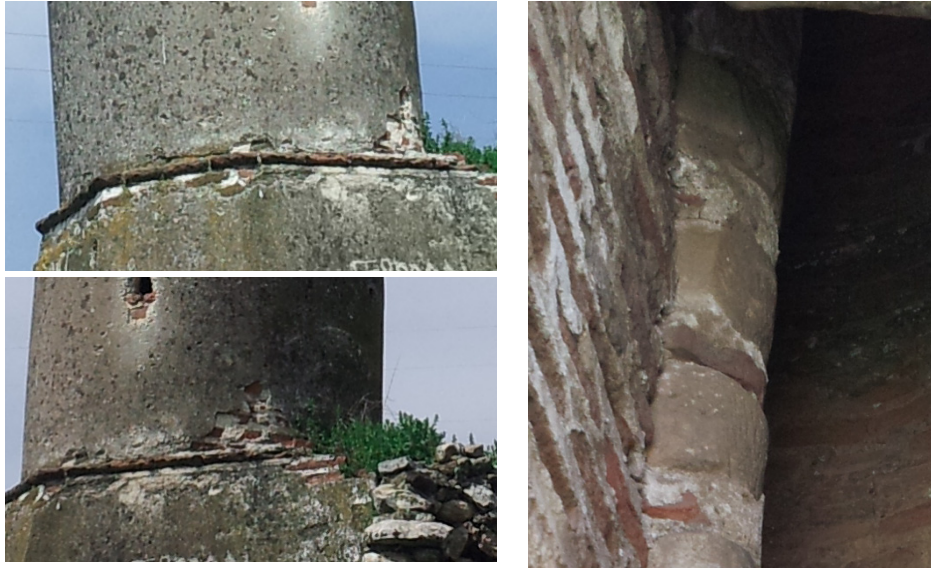
Figure 21. Existing cracks and damages on the minaret
