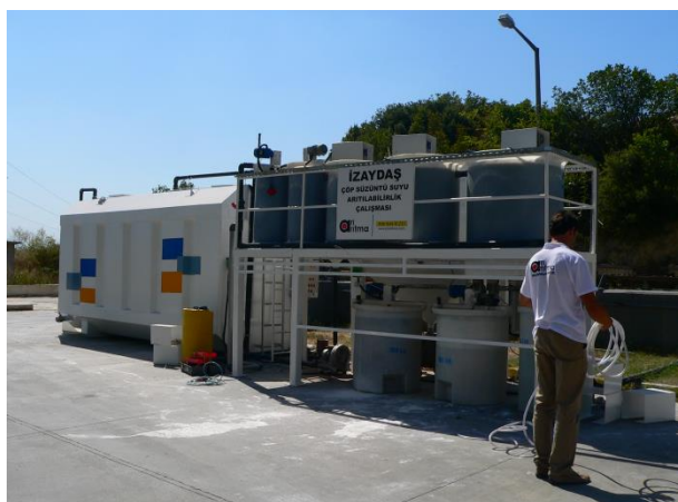
Figure 2. Biological-chemical treatment prototype facility appearance
