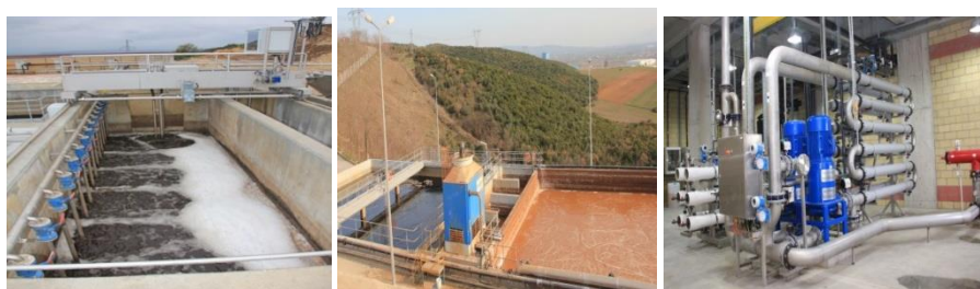
Aerated sand-oil trapping balancing and biological pools UF membranes
