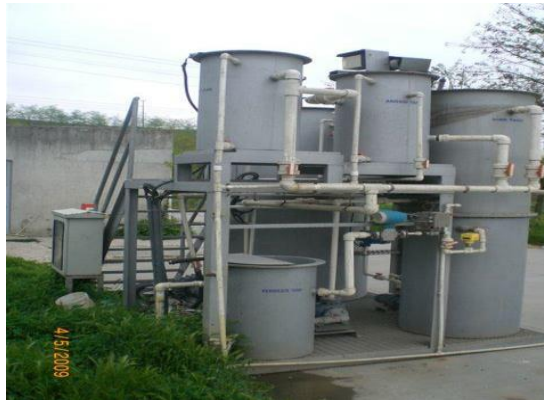
Figure 5. MBR Prototype Facility General Appearance
