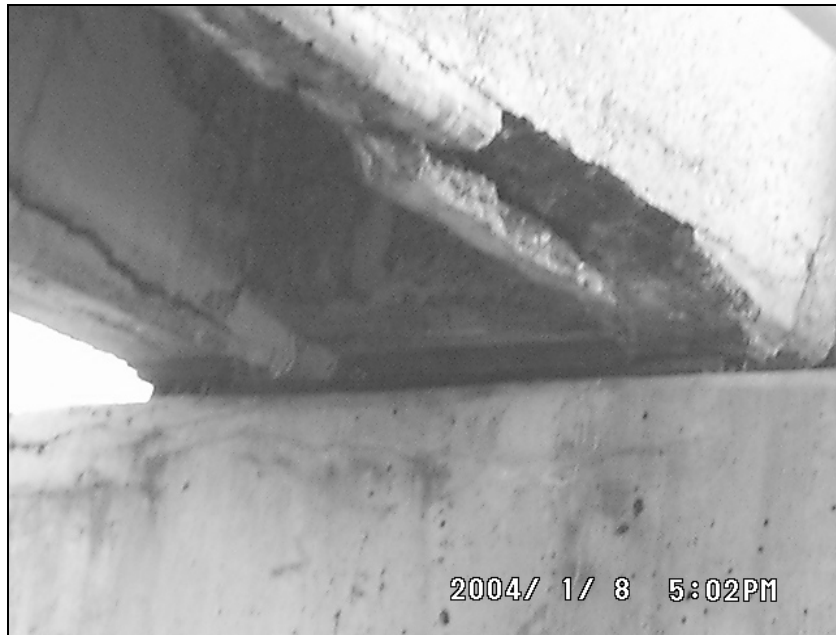
Fig. 6. Separation of concrete at beam faces
