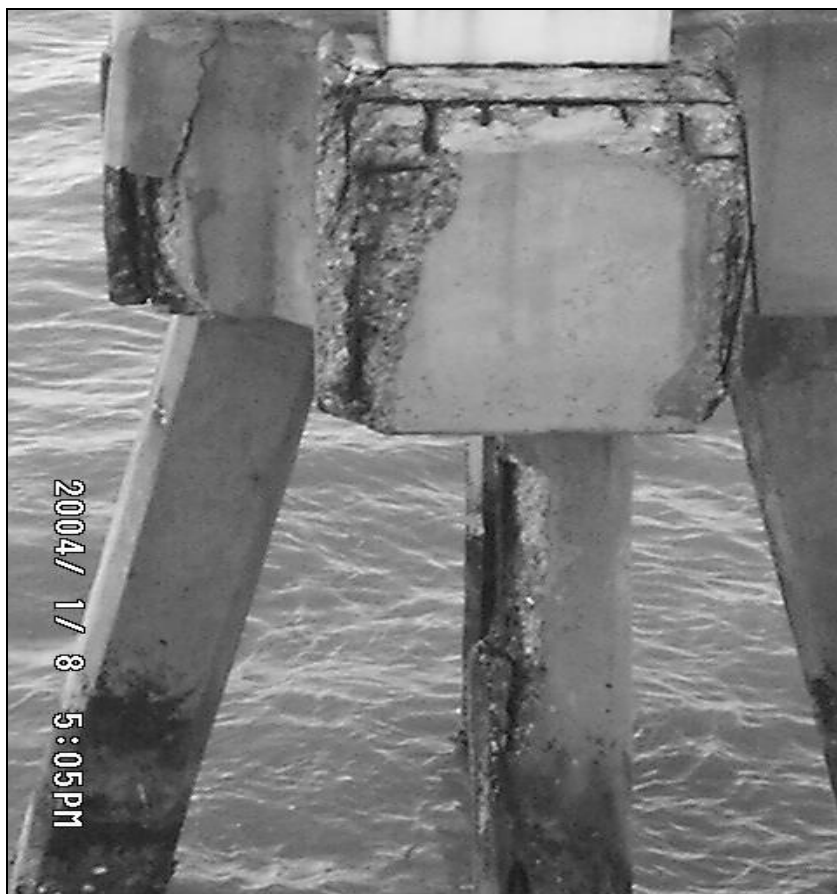
Fig. 12. Corrosion in RC piles
