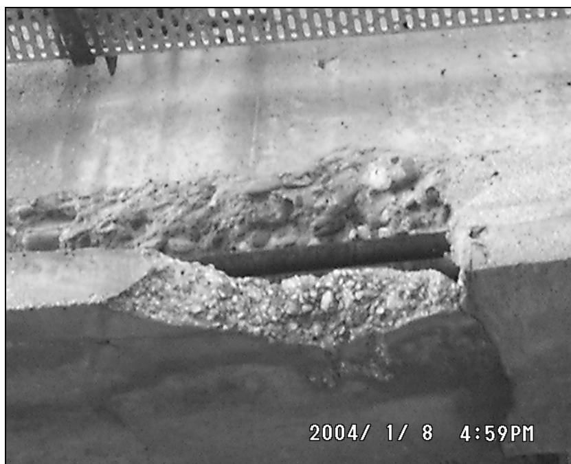
Fig. 5. Concrete damage at beam faces.
