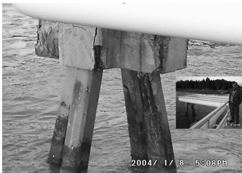
Fig. 9. Corrosion and structural damage in RC piles
