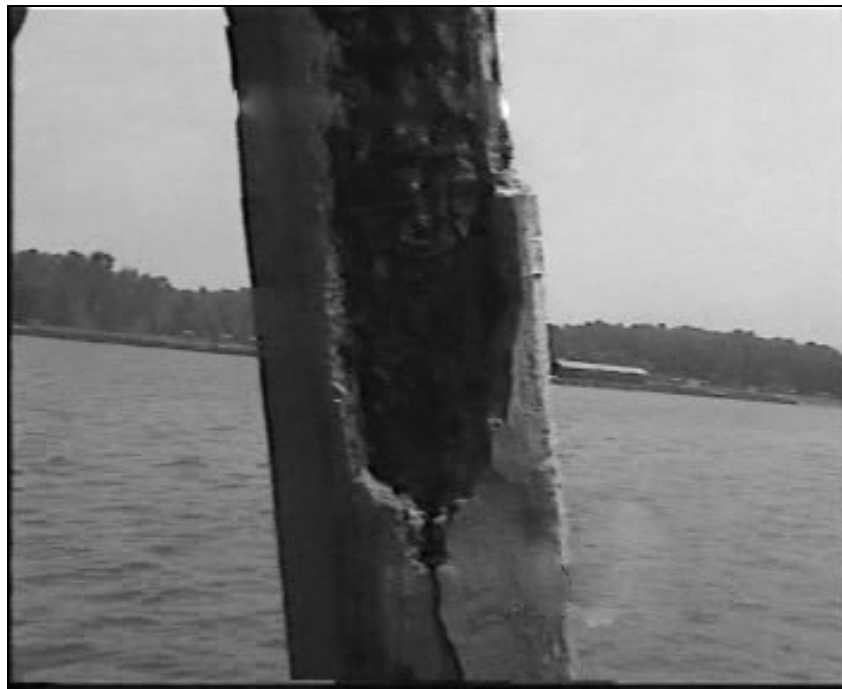
Fig. 11. Cover of concrete has fallen and the reinforcement is corroded heavily.
