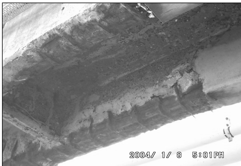
Fig. 13. Corrosion in RC beams
