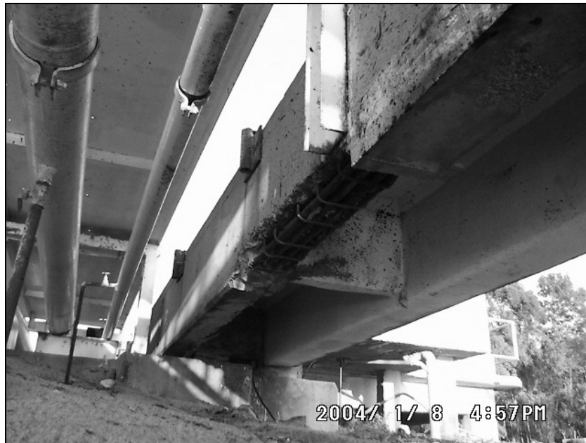
Fig. 3. Some damages in a beam
