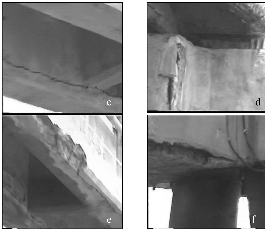
Fig. 8. Corrosion and structural damage in RC piles near to sea surface a) Damage in two piles. b) Concrete fall down and reinforcement corroded. c) Longitudinal cracks in a beam. d, e & f) Serious damages in beams
