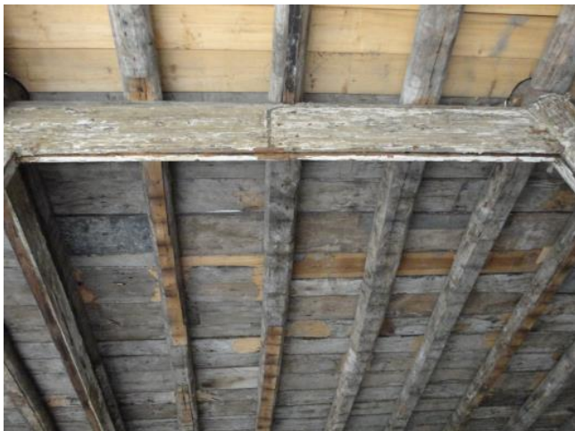
Figure 1. Cracks in square beam
