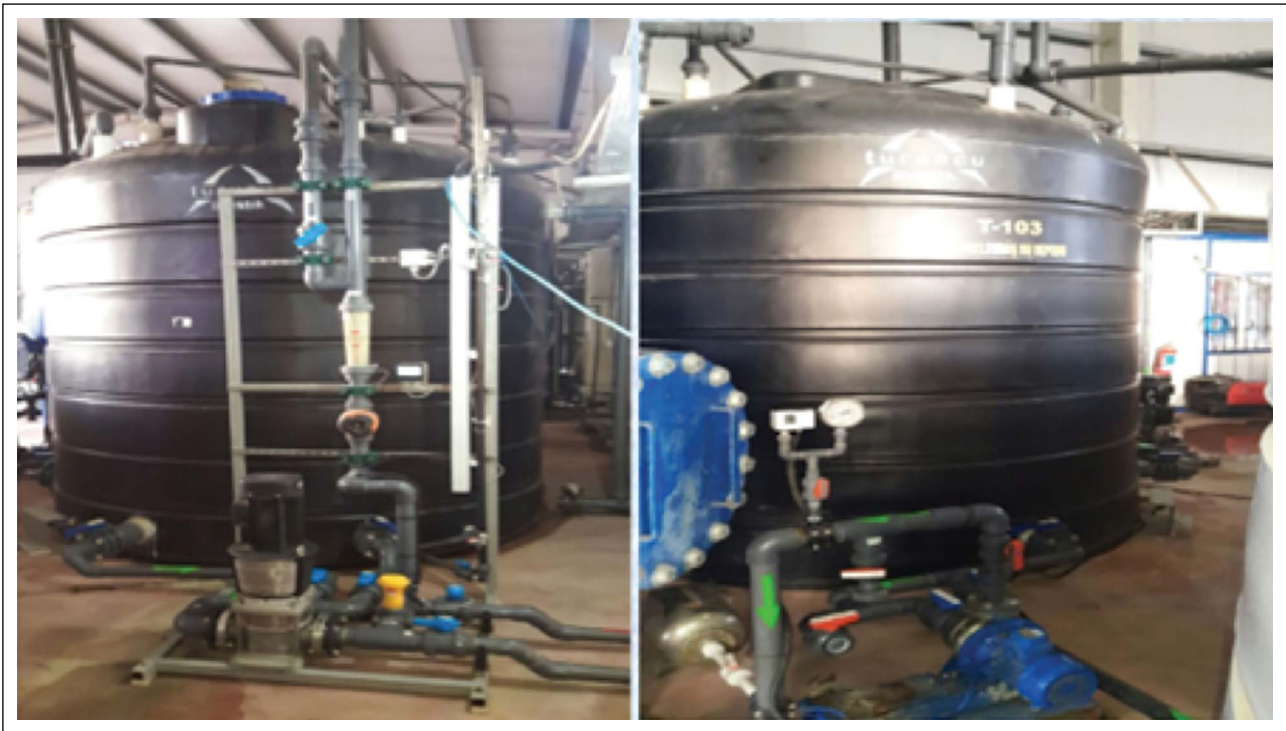
Figure 5. Tank 3 for pH adjustment.
