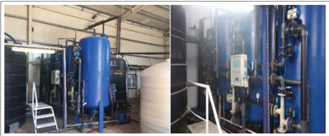
Figure 4. Sand filters in the system.
