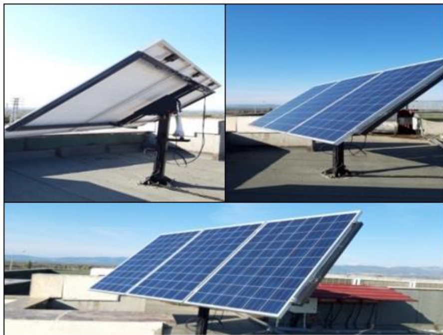
Figure 10. View of Solar Power Plant-2
