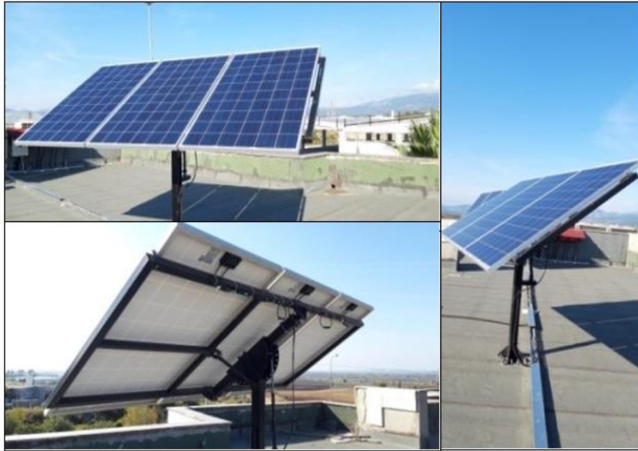
Figure 8. View of Solar Power Plant-1
