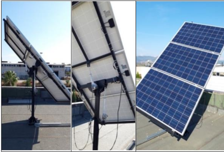
Figure 12. View of Solar Power Plant-3
