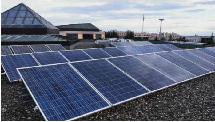
Figure 2. The PV panels on Kocaeli University Technology Faculty building
