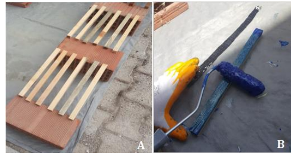
Figure 1 Image of the wrapping process with FRP polymers, A: Preparing the beams for wrapping after the priming process B: Wrapping the beams with FRP polymer fabric
