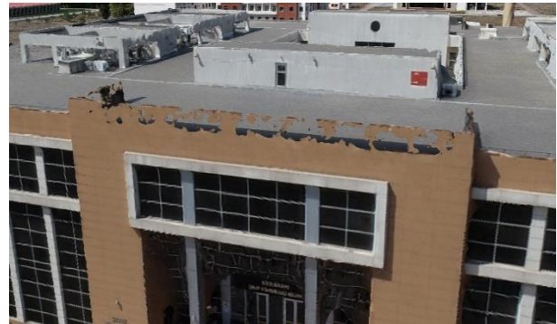
Fig. 14. Gaps on building rooftop surroundings
