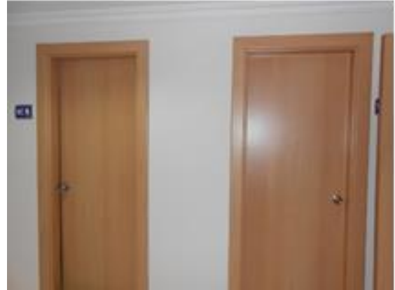
Figure 11. Emergency department waiting room water closets of sample B
