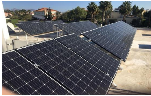
Figure 19: Solar panels on the flat roof (Author, N.U)
