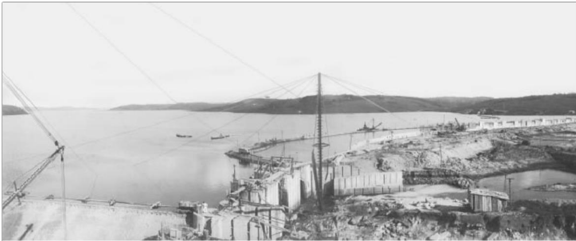
Figure 1 – Construction of Pedreira Dam at the Rio Grande water course in 1928. Source: Capobianco & Whately (2002).
